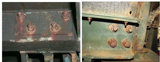
Figure 28: MTRV Truck Frame Fastener Corrosion
