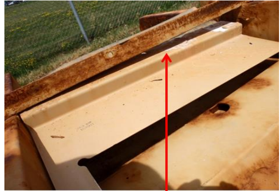
Figure 17: Location of Water Trap associated with the FMTV Auxiliary Transmission Cooler Shroud.
