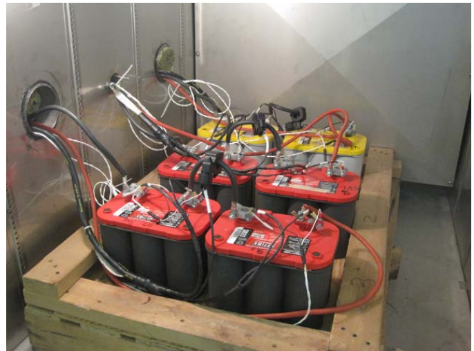
Figure 6: Batteries Installed In Chamber
